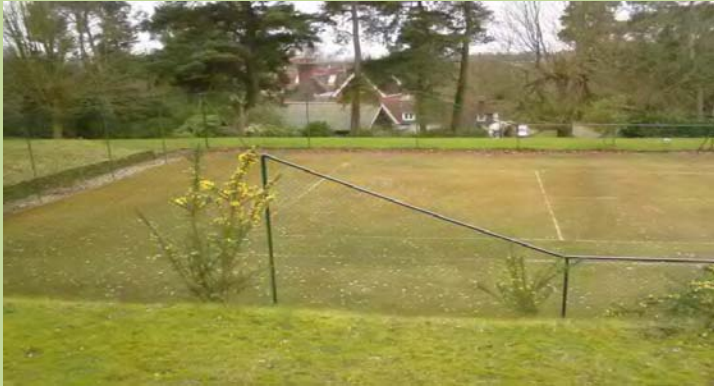
Tennis court contaminated by moss & algae before Rejuvenation
