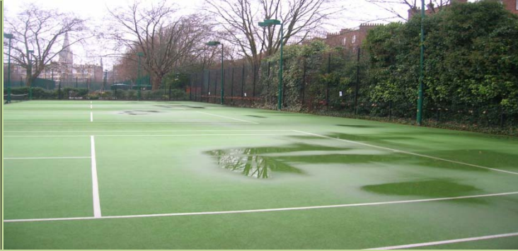
Infill compaction & contamination leads to flooding and poor drainage
